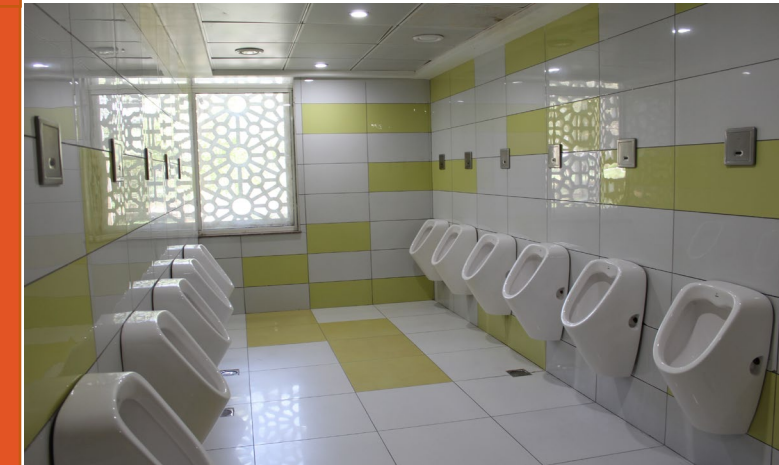
Smart Toilets based on urinal sensors
